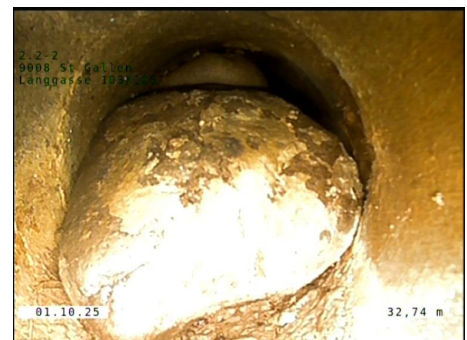
Pos: 12 - 12; Lose Ablagerungen, Kies, Höhe = 80%, Grosse Steine in Fallrohr
