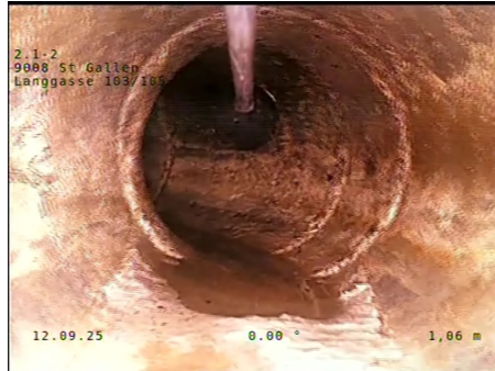
Pos: 6; Harte Ablagerungen, Höhe = 0%
